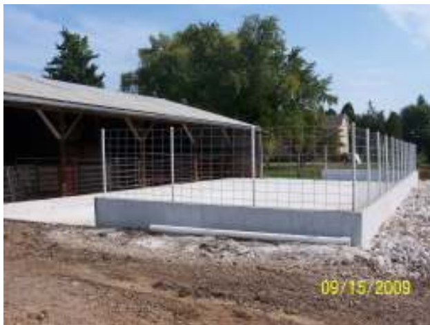
Above: Barnyard installed to control animal waste through EQIP
